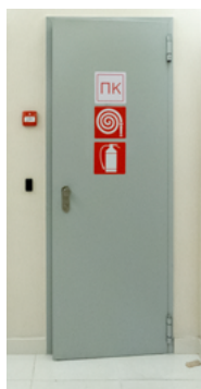
Fire hose cabinet
