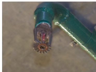
Sprinkler in the garage
