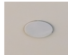
Sprinkler in the office
